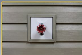
Hose bibs, sumps, gas lines, vacuum lines
